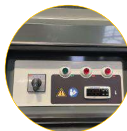
Panel de control
